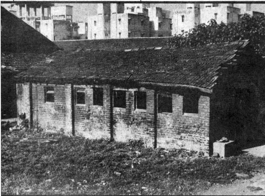
Shoddy and dilapidated toilets: Worli police lines.
